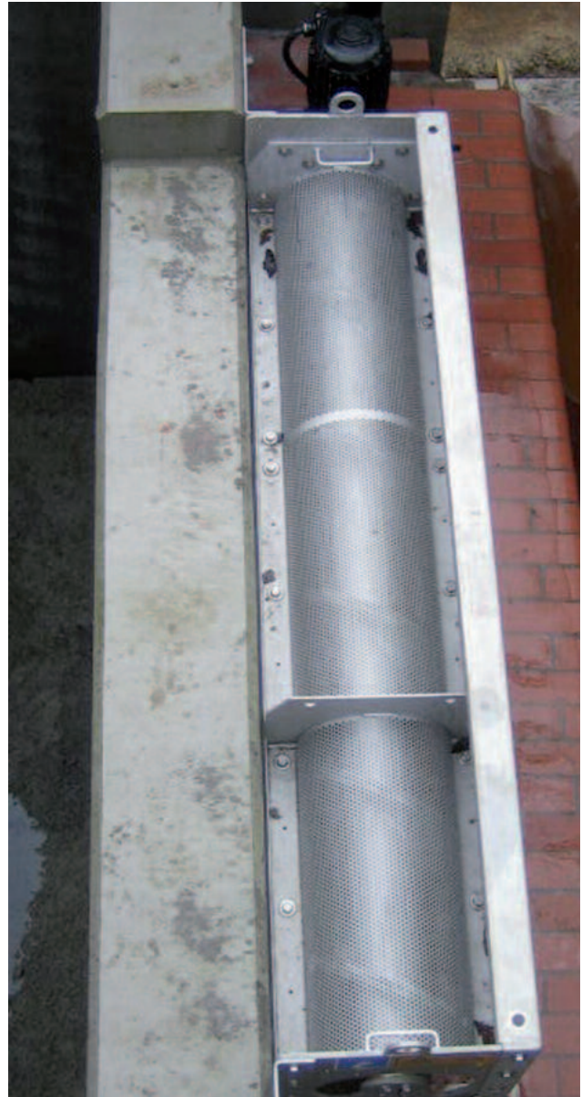
ROTAMAT® Storm Screen RoK 2 installed at a stormwater discharge
