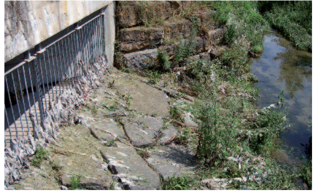
Unsightly matter discharged during storm events, typical for stormwater discharges without coarse material retention
