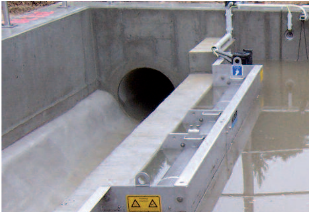
HUBER ROTAMAT® Storm Screen RoK 2 before overflow
